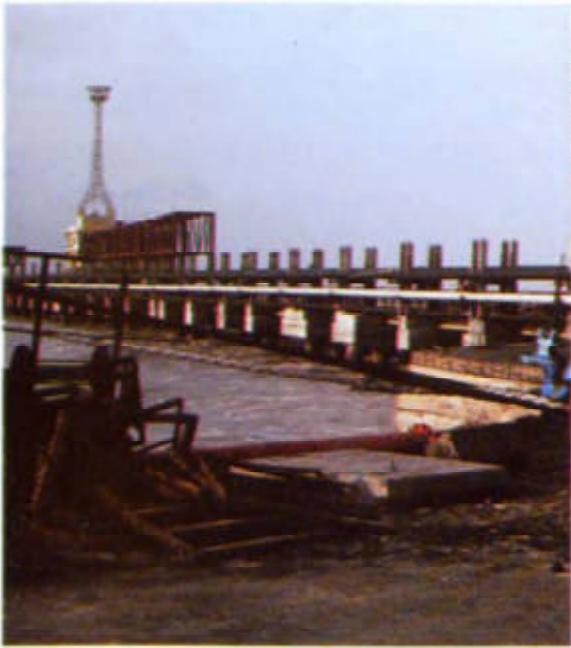
Construction activities of Mundra Port, for crude oil pipe line in the coastal regulatory zone
